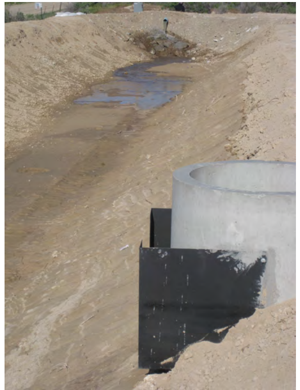
Figures 5A and 5B - Cipolletti Weir at the Outlet of the Sedimentation Basin
